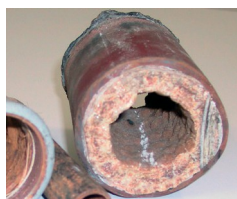
Hard water is a threat to boilers - it also causes a significant reduction in the thermal efficiency of the heating system.
